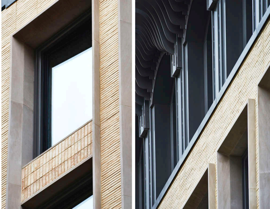
Close look at the beautiful brick and metal work of 150 Wooster (KUB)
