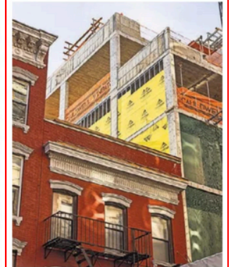
Above left and center, 214 West 80th Street, which was bought by Terra Developers. Above right, a parking garage on East Ninth Street in the East Village, which was bought by the real estate developer Arcus.
